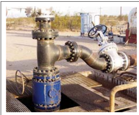
Master Valve Geothermal Brine
