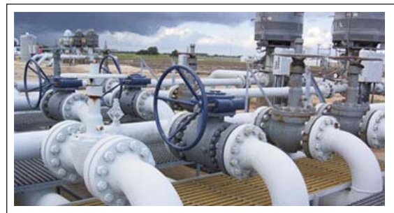
Salt Dome Brine & Gas Pumping Station
