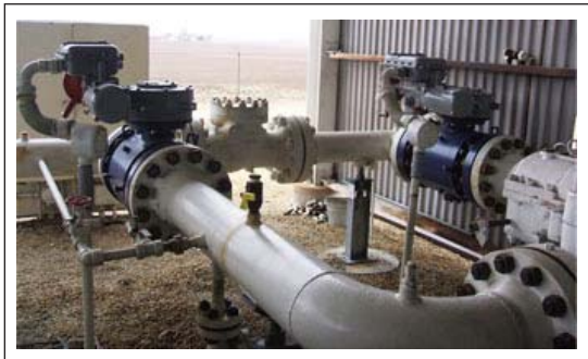
Crude Oil Pumping Station Pig Launcher/Receiver
